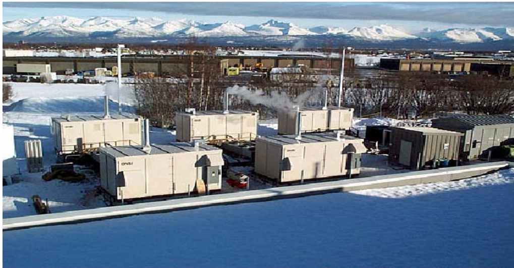
U.S. Postal Service in Alaska 5 – PC25 (200 kW) Power Plants International Fuel Cells
